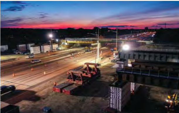
The Tollway is reconstructing the Burlington Northern Santa Fe (BNSF) Railway Bridge over I-294 near Hinsdale and Western Springs to accommodate widening of the Central Tri-State Tollway (I-294).
