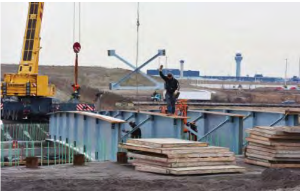
Beams are placed to construct the I-490/Illinois Route 390 Tollway Interchange near Bensenville.
