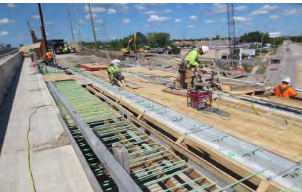
Crews are reconstructing the Edens Spur Tollway (I-94) from Pflugsten Road to the Edens Expressway near Northbrook to extend the life of the roadway and provide safe travel for Tollway customers.
