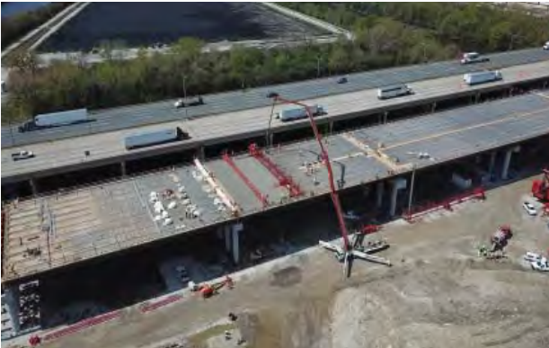
Concrete is poured to construct the new I-294 Mile Long Bridge near Willow Springs as part of the Central Tri-State Tollway (I-294) Project.
