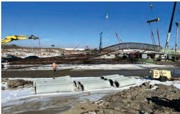
Shafts are assembled to connect the new I-490 Tollway with the Jane Addams Memorial Tollway (I-90) Interchange near Des Plaines.
