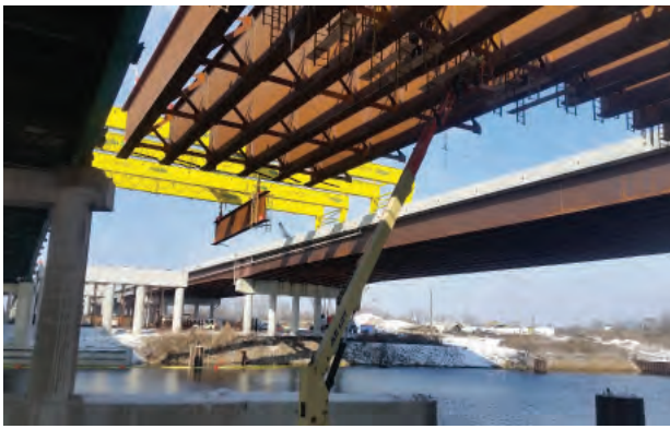
Beams are placed over the Chicago Sanitary and Ship Canal for the new southbound Mile Long Bridge along the Central Tri-State Tollway (I-294) near Willow Springs.
