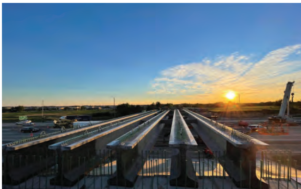
Beam placement has begun along the Central Tri-State Tollway (I-294) for the new Stearns School Road Bridge near Gurnee. The new bridge will provide for three lanes of traffic and replace a 70-year old structure.
