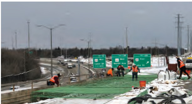
Roadway and bridge reconstruction continues along the Central Tri-State Tollway (I-294) near Elmhurst.
